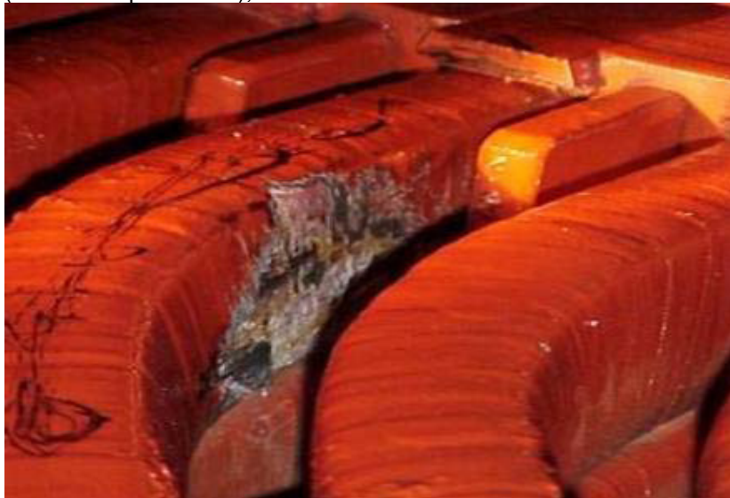
Picture 10: Insulation failure in end winding
