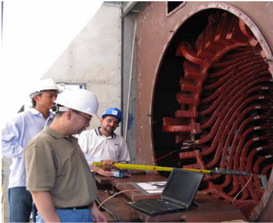
Picture 12: Off-line PD test with Corona probe
