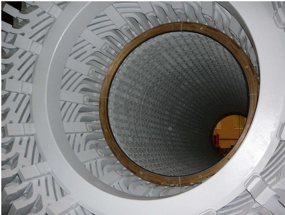
Picture 1b: Stator end winding support structure of Air-cooled generator
