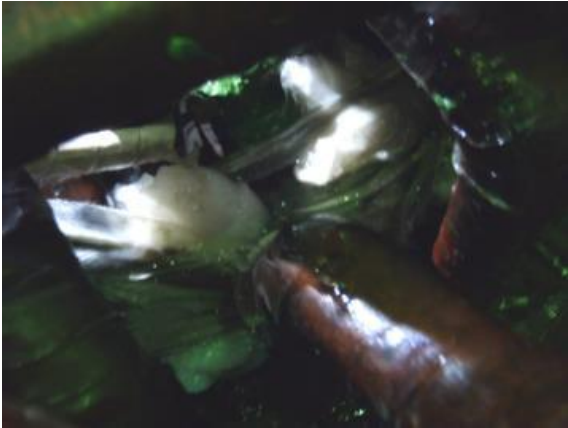
Felt and fibreglass tape behind coil #35.
