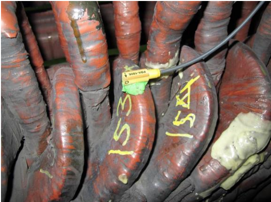
FOA-100E optical accelerometer on an end winding
