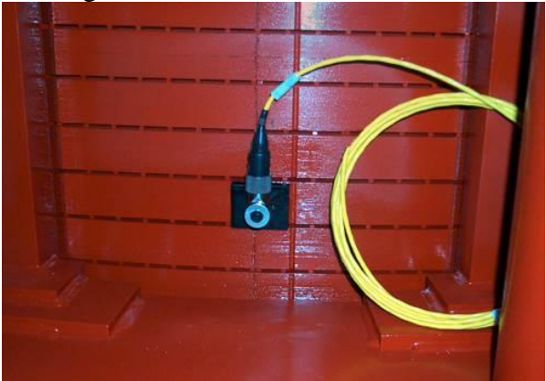
Accelerometer on stator core (Example only)
