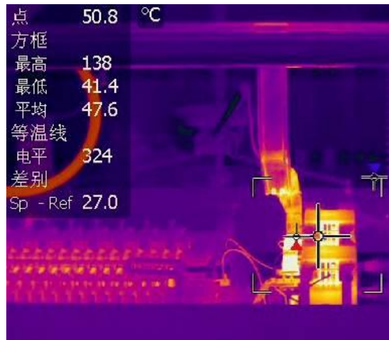
Fig. 15 The overheat of the valve reactor connectors
