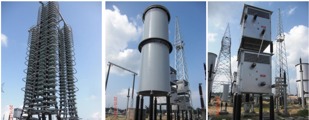
Figure 3 – DC filter high-voltage capacitors, reactors and resistors at Biswanath Chariali
