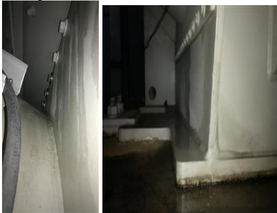
Fig. 14a 800kV converter transformer Oil leakage
