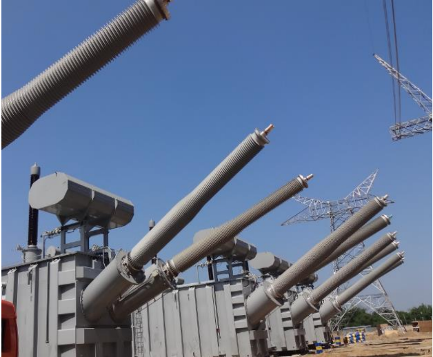
Fig-4 800 kV Converter Transformer of NER-Agra HVDC Project (under construction).
