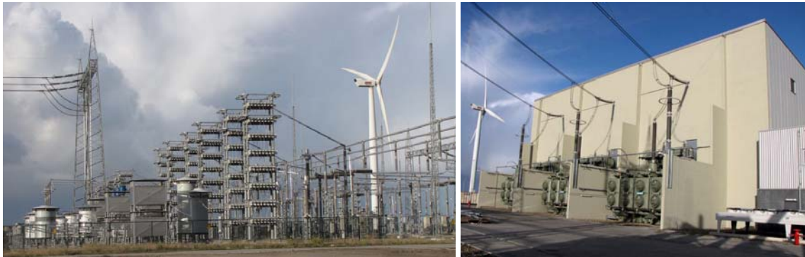
Fig. 2: Line-commutated converter station in operation
