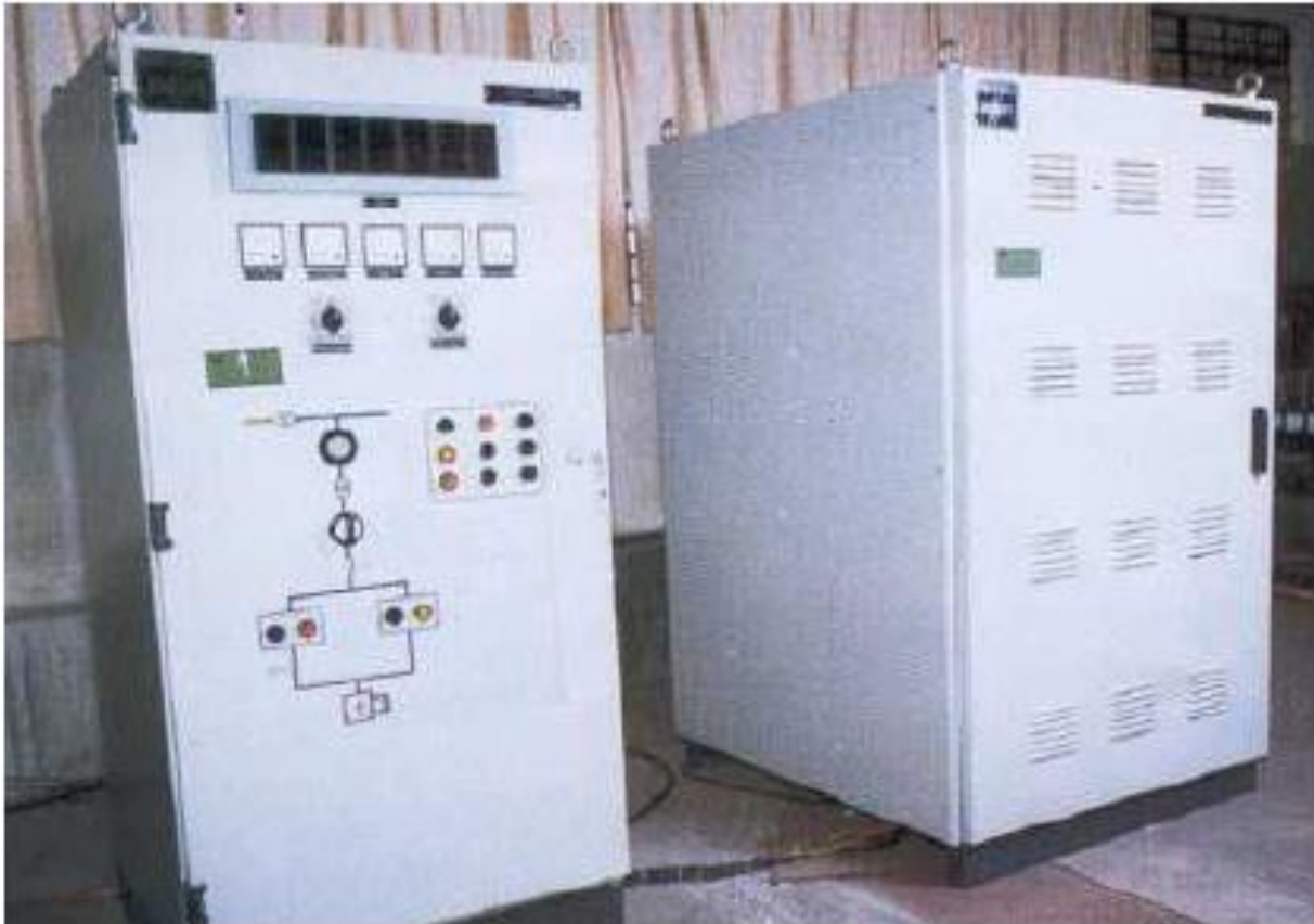
Figure-5: Photograph of IGBT power and controller panels for \pm 500 Kvar D-STATCOM
