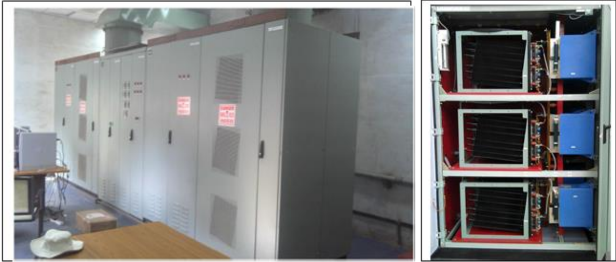
Figure-10: A view of the installed STATCOM at Foundry shop of BSP
