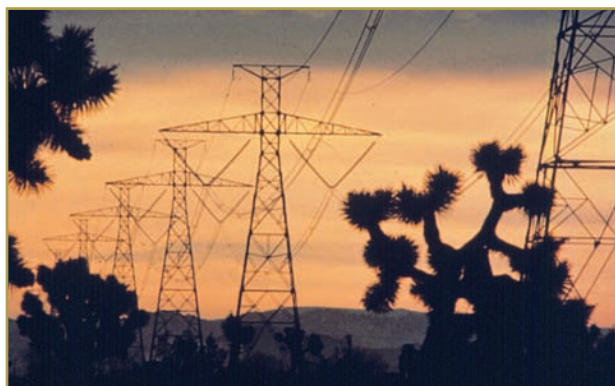
figure 2. A ±500-kV HVDC transmission line.
