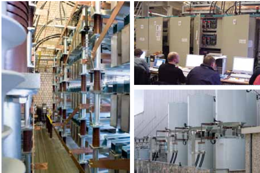
Fig. 22: 30 MW Hardware Functional Tests
