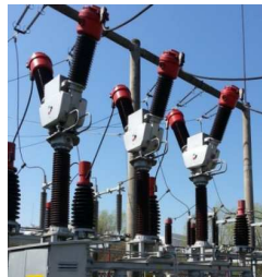
110kV High voltage breaker picture
