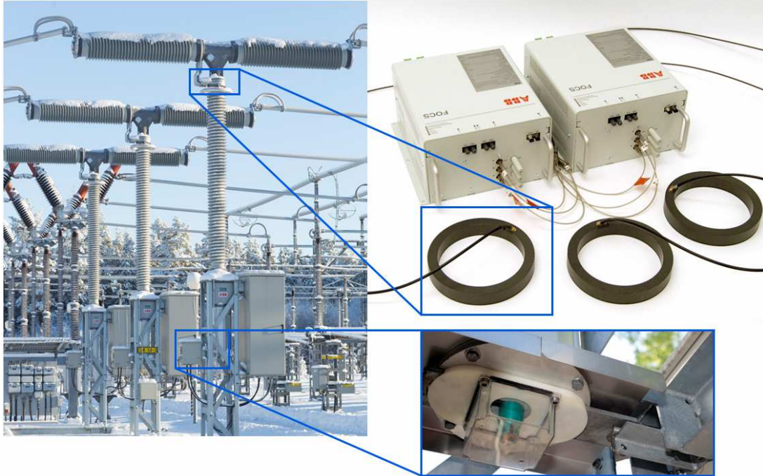
Figure 4: (Left) Pilot installation of a combined unit DCB with NCIT's of fiber optical current sensor (FOCS) type. (Right above) three phase FOCS-kit with three sensor heads and two opto-electric modules for redundancy. (Right below) One type of mechanical locking system for DCB as required by the IEC 62271-108 standard.
